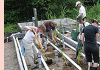
Staff from Fleming's Centre for Alternative Wastewater Treatment completing a research project.
